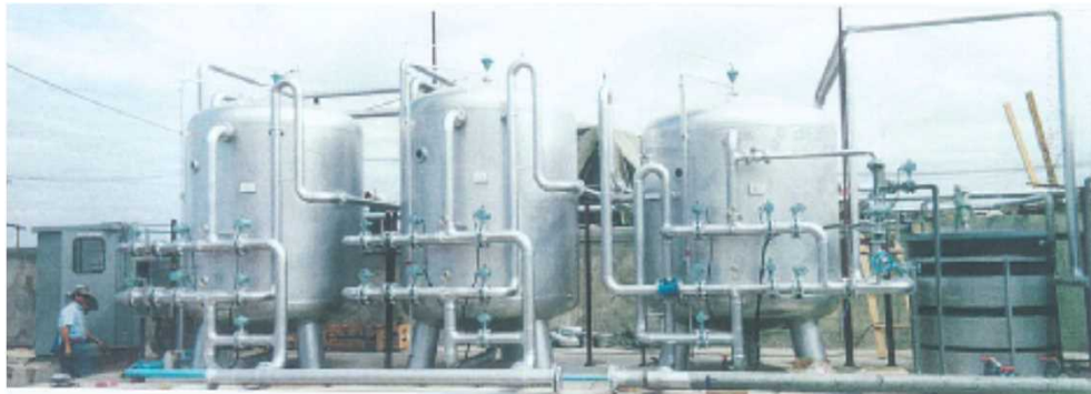
Rapid Filter + Softener (River Water Treatment)
