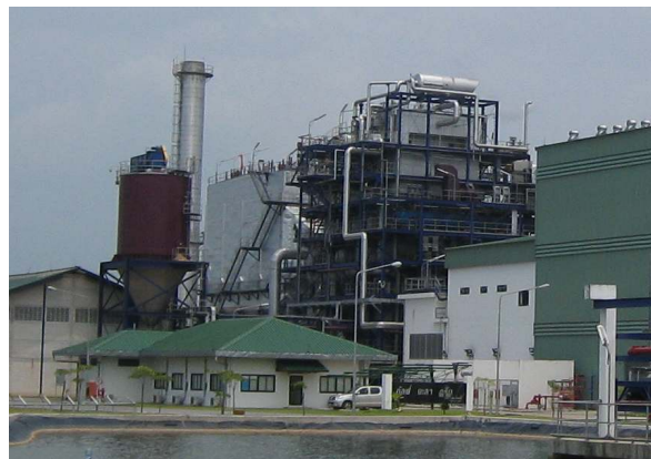
Rubber Wood Fired Boiler Plant Thailand 23,000 kW
