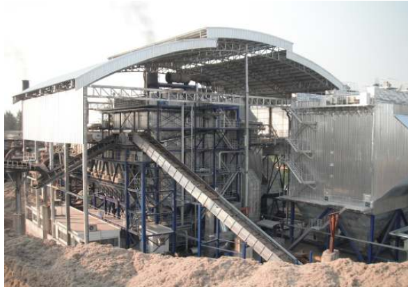
Bagasse Fired Boiler Plant Thailand
