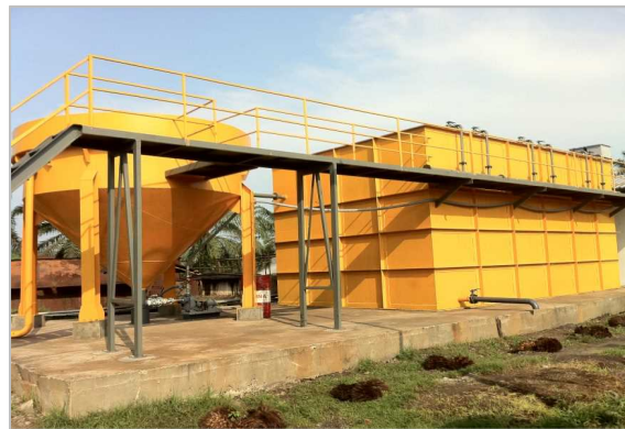
Indonesia P Palm Oil factory ,Ministry of the Environment co-benefits environmental technologies Japan - Indonesia bilateral cooperation projects 2014 by Aerator 12 sets
