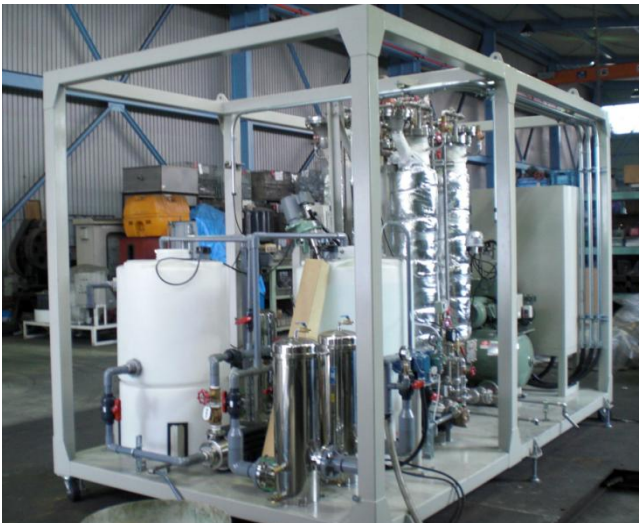
[Effluent purification system (medium size)] (treatment capacity: 10 t/day)
