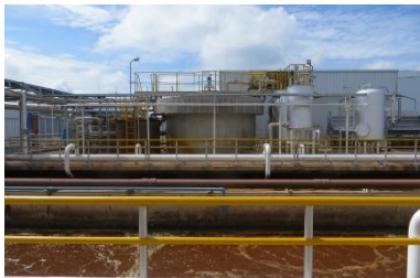
Wastewater treatment facility Dyeing factory (Thailand) Capacity: 800m 3 / day
