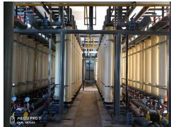
Sewage treatment facility (China) Capacity : 15,000m 3 / day
