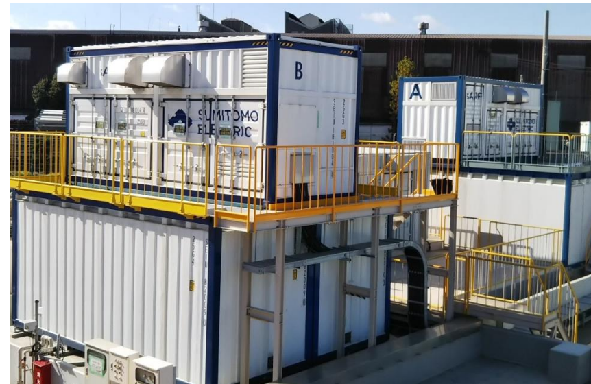
Location: Sumitomo Electric, Osaka Works Capacity : 750kWh (250kW × 3h)
