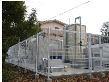
Well water purification system (Hospital)
