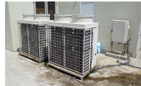
Saving-Energy, Spraying water system (Hotel)
