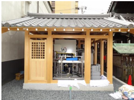
Well water purification system (Shrine)
