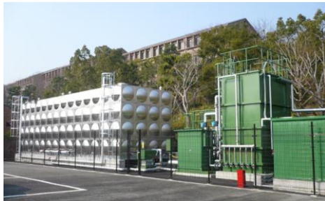
Well water purification system (University)
