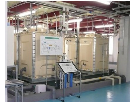
Reuse water treatment system (Building)
