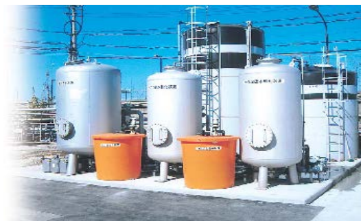
Full automatic well water treatment (Deferrization & Demanganization + Softener)
