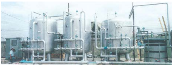
Rapid Filter + Softener (River Water treatment)
