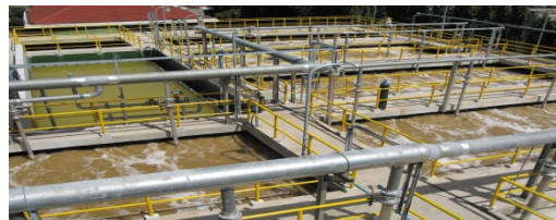
Wastewater treatment (High salt concentration waste water treatment by the halophilic microorganisms)
