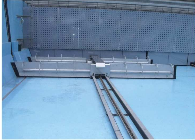
Unit delivered to a water treatment plant
