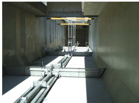
Monorail sludge scraper
