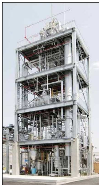
Solvent recovery equipment
